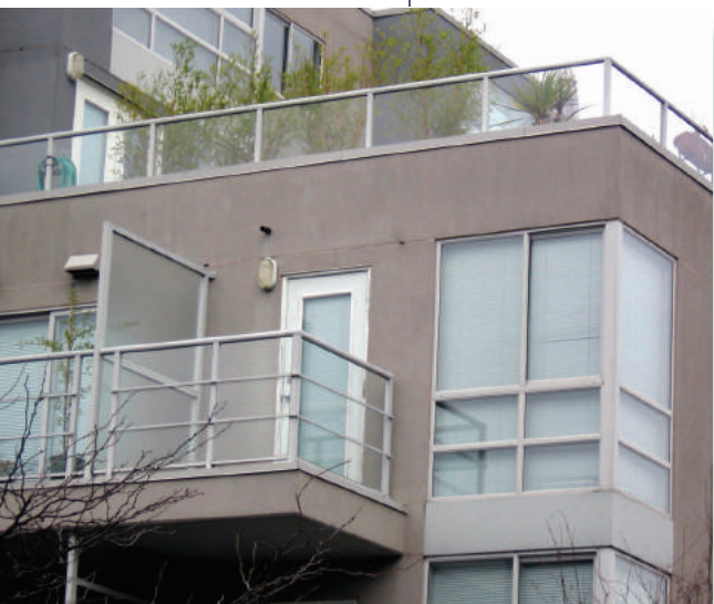
Windows and exterior doors deteriorate over time due to age, wear and tear and the weather, and require ongoing inspection and maintenance.
